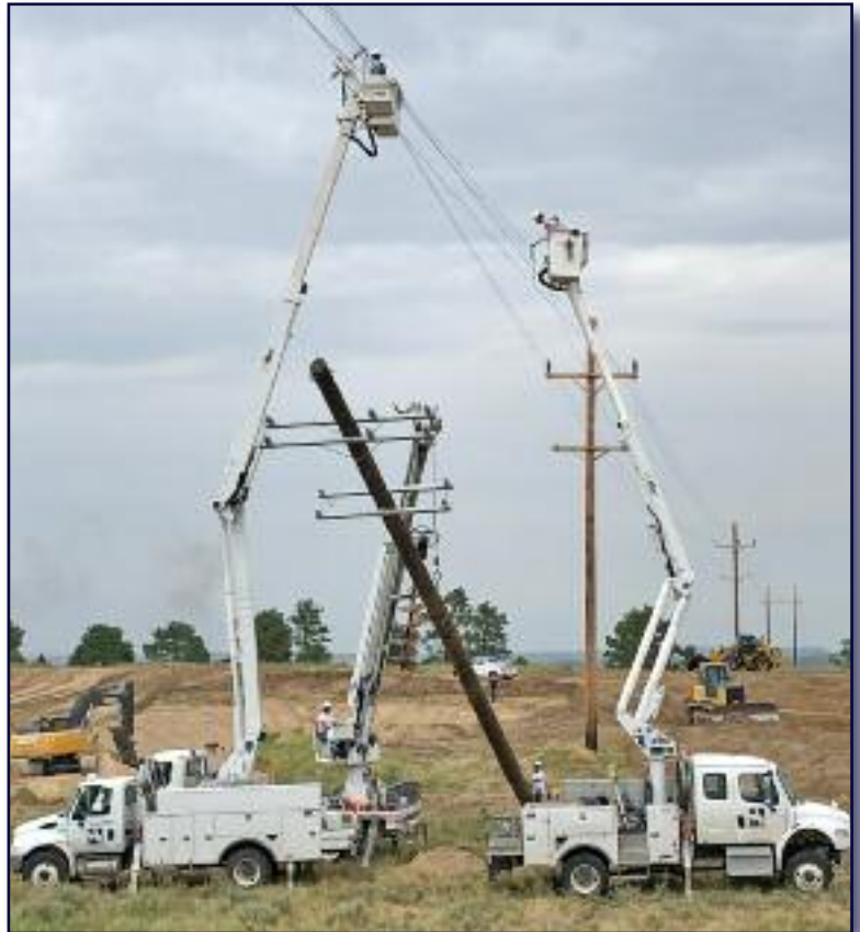
Wyrulec crews work to set a new 75 ft. transmission pole near the area where the tunnel collapsed.
